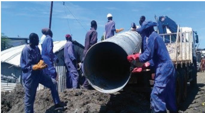
IOM CCCM Care and Maintenance casual labors installing a new culvert in the Malakal PoC site © IOM CCCM 2021
