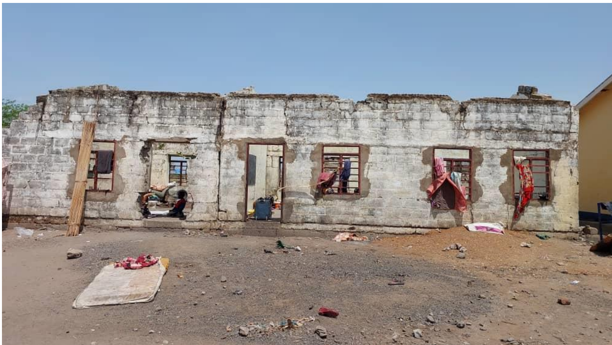
Figure 1: One of the school classrooms without roof and doors being used by the returnees for shelter at Abukhadra primary school.
